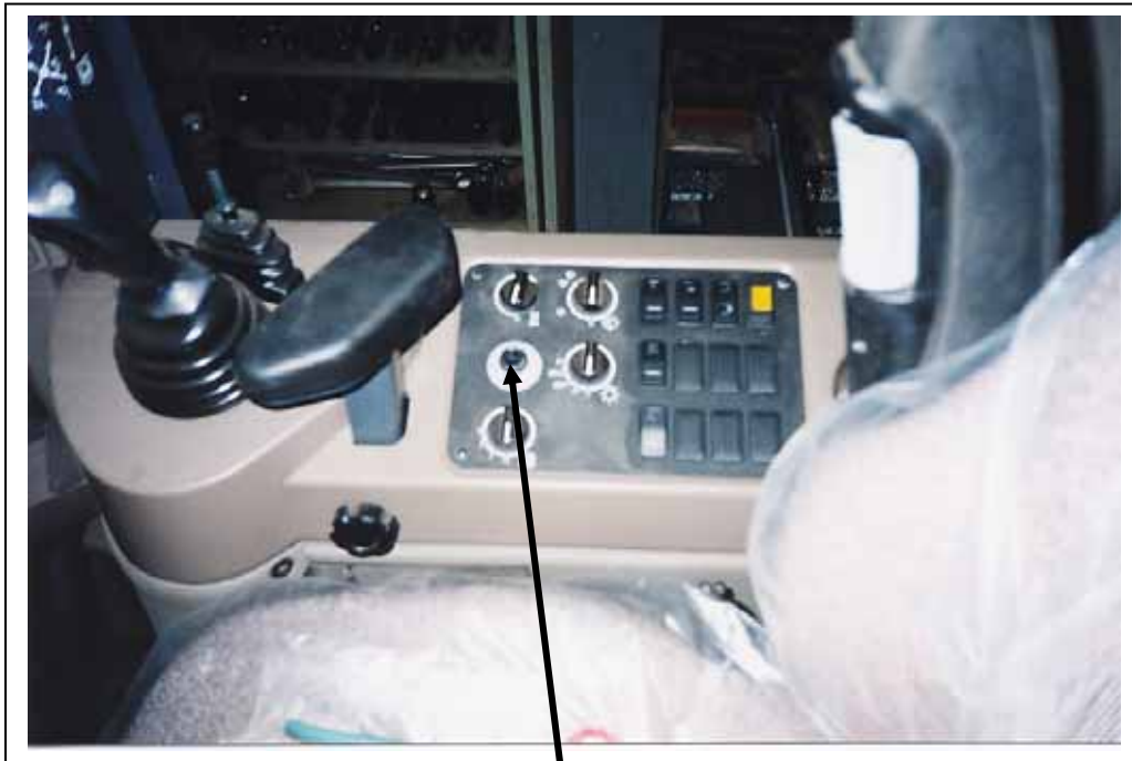
Thermostat location in cab on right control panel
